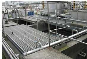
Drainage handling facility
